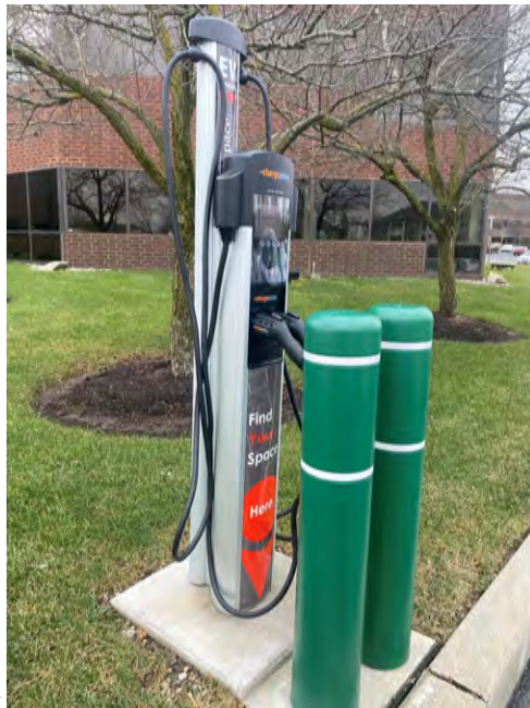
Electric Car Charging on site
