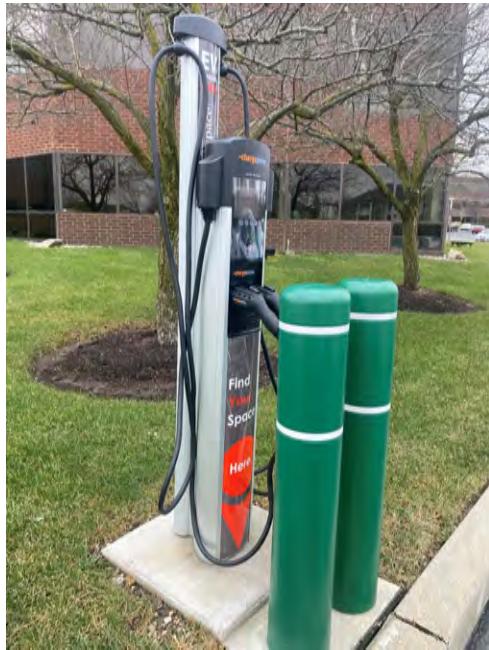
Electric Car Charging on site
